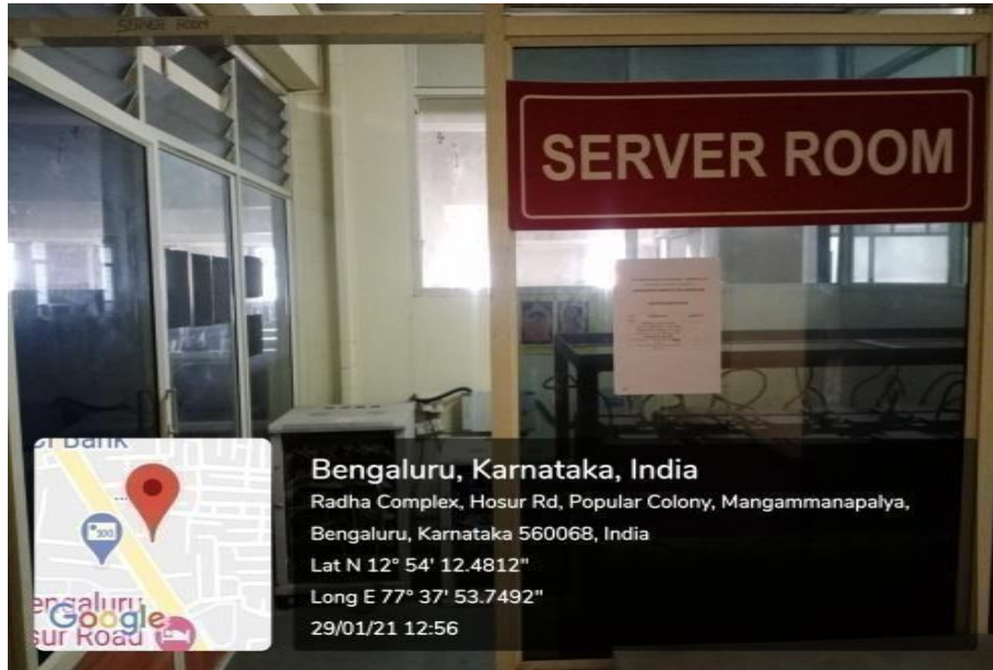
List of ICT Facilities available in the R&D Center
